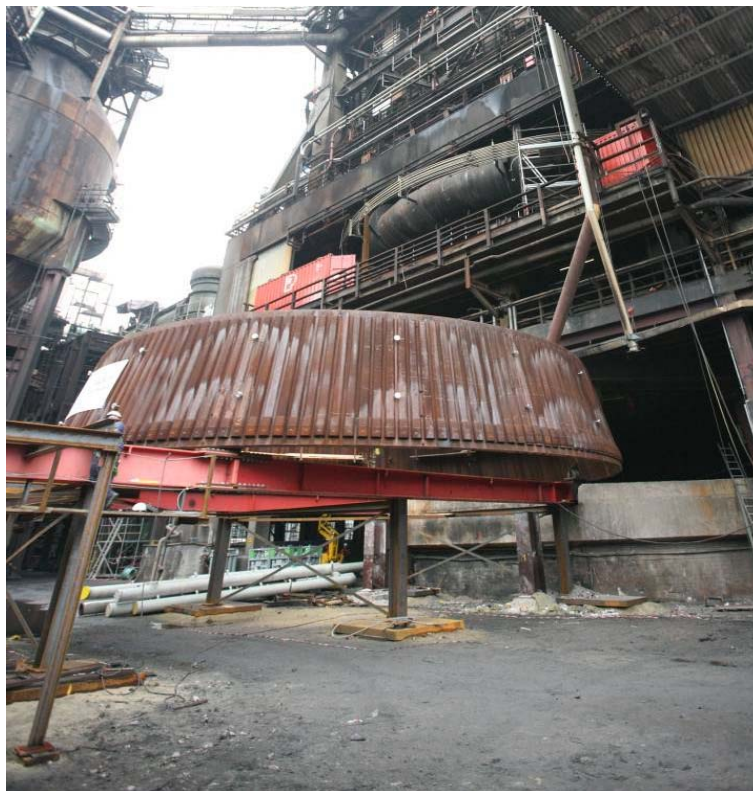
Figure 4. Displacement of a ring element of the hearth shell on the slide rail.
