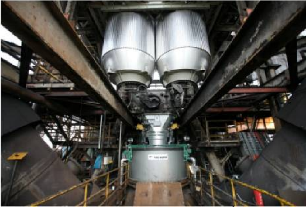
Figure 7. Shows the new hoppers and the Paul Wurth BLT ® GEN3 gearbox
