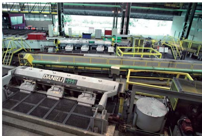
Figure 2. Arrangement of twin DWB high-speed finishing blocks
