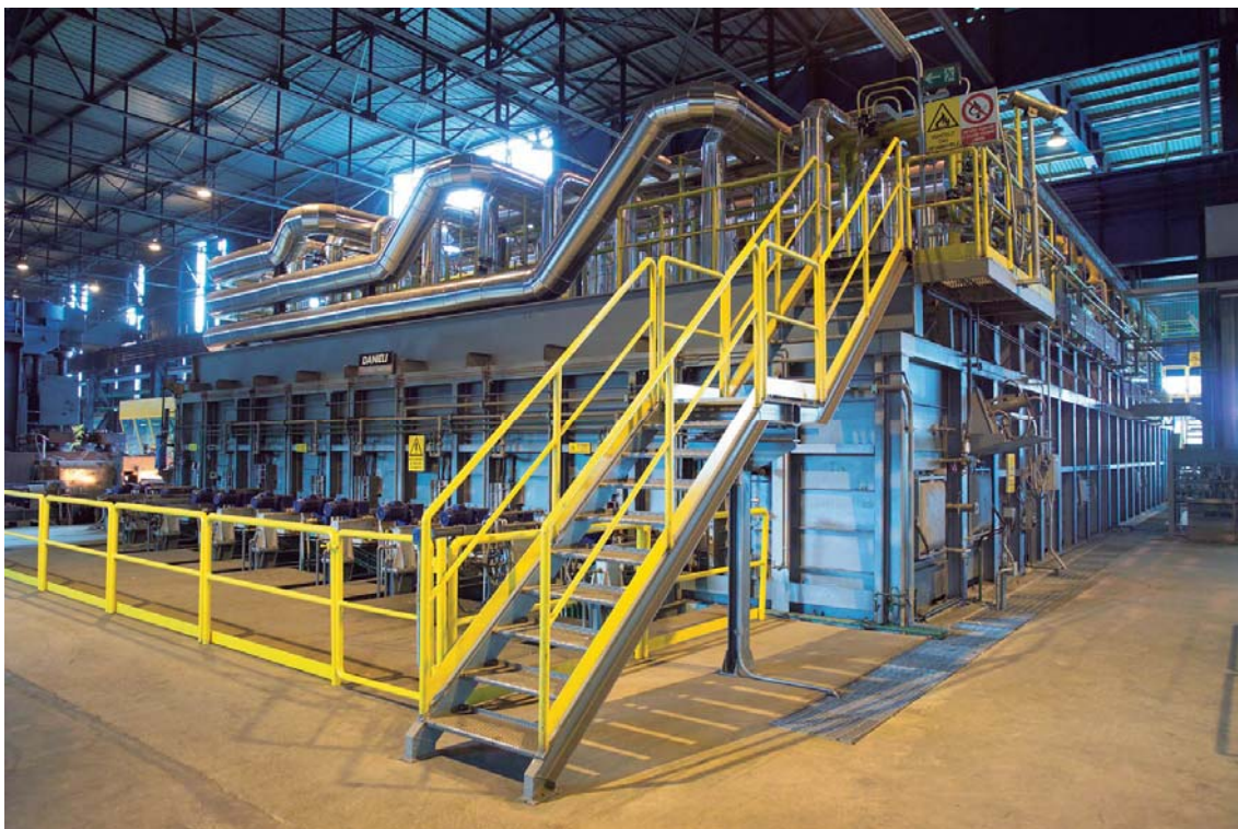
Figure 1. WB Furnace in Operation – Ferriere Nord – Osoppo (UD) – Italy.
