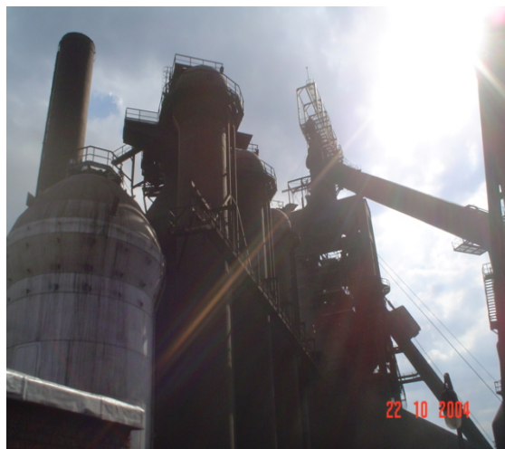
Figure 1 – Mittal SA Vanderbijlpark BF D – Fourth Stove
