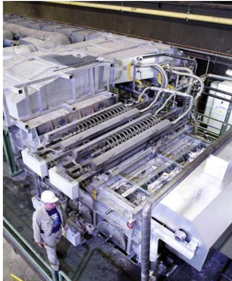
Figure 3. The DFI Oxyfuel unit installed at Finnentrop, replacing part of the dark-zone and boosting the output by 30%.
