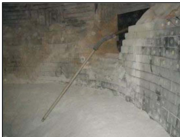
Figure 9. Probe position in empty furnace.
