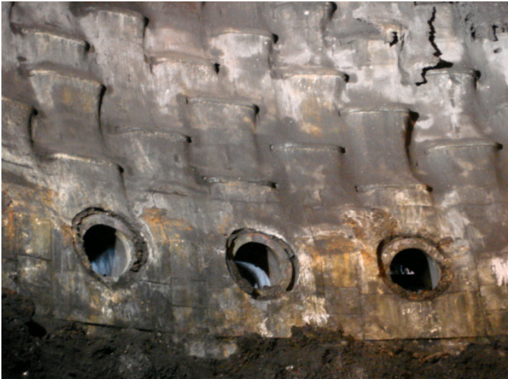
Figure 2. Limited wear after ten years in operation (plate cooled bosh).
