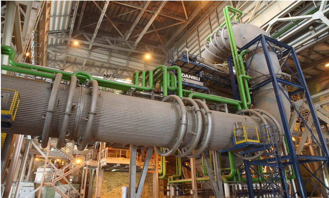
Figure 3. Cooled fume duct system.
