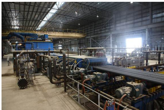
Fig. 8: Spray Box at Shotblaster Entry Side
