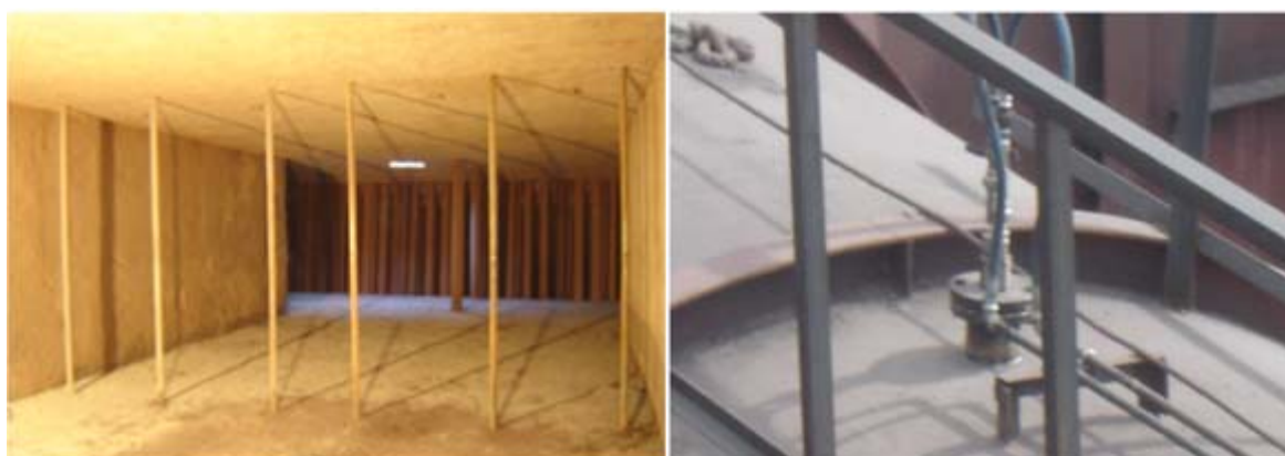
Figure 6 - Pitot tubes inside / outside the ductwork
