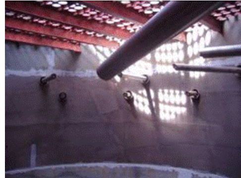
Figure 12: Water injection lances
