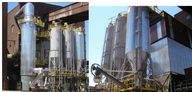
Figure 13: Demonstration plant at voestalpine
