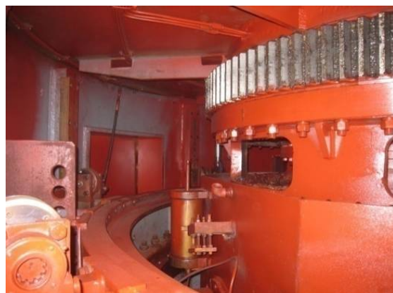
Figure 3. Interior structure of BCQ distributor.
