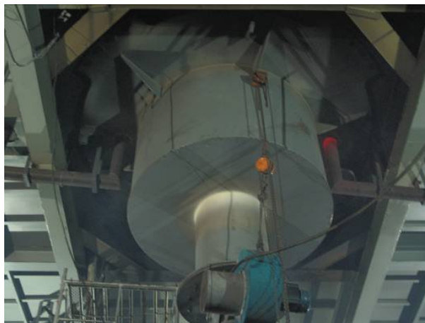
Figure 7. Hot test for distributor.
