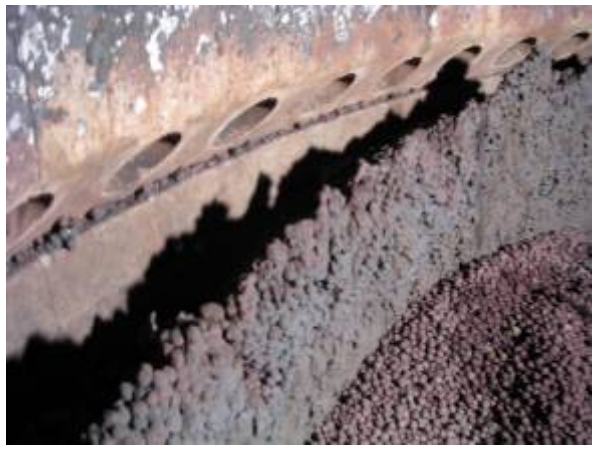
Flagstone clusters separated from the wall to remove and clean the nozzles.
