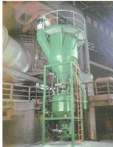
Figure 5. Injection system and silo for Synthetic \text{TiO}_2 products.
