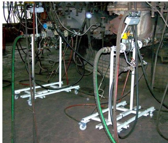
Figure 6. Injection lances for RUTILIT Products at the blast furnace.
