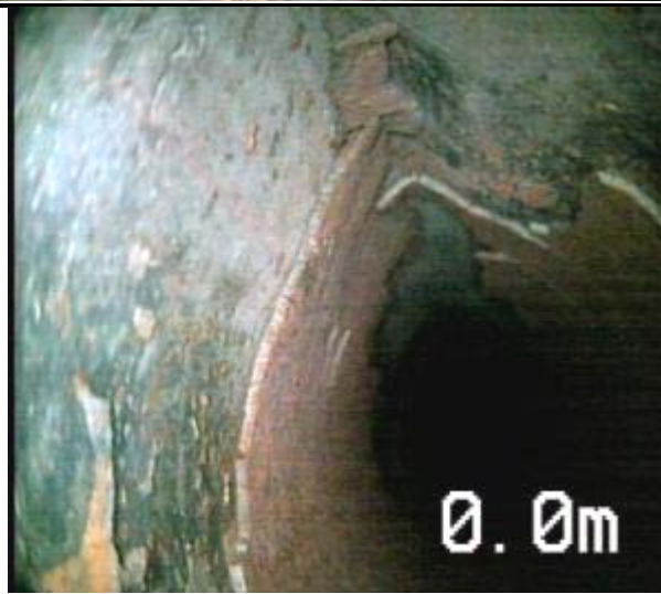
Inside view of cooling staves tubing showing piping damages
