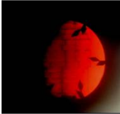
Figure 2 – Aspect of Dividing Wall Cracks in # 1, 2 and 3 Hot Blast Stoves Combustion Chamber
