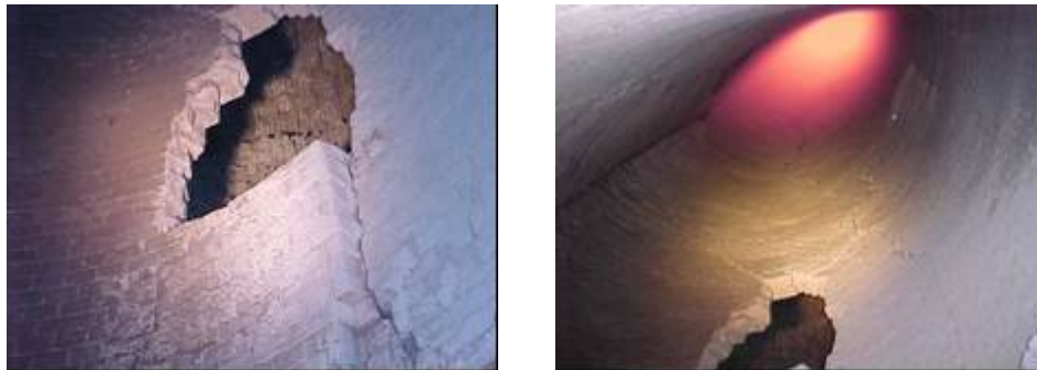
Figure 1 – Dividing Wall Breaking Open and Checker Bricks Caving In at Combustion Chamber Bottom of Hot Blast Stove # 3, 2002.
