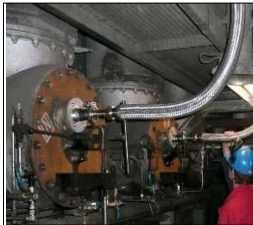
Figure 3. Burner Installation at SSAB
