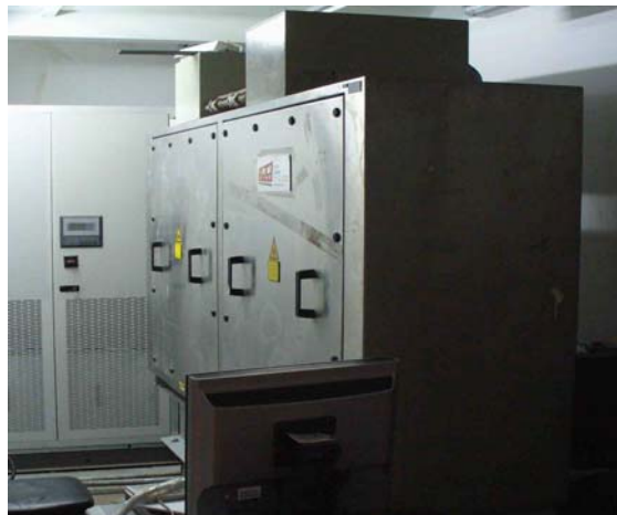
Figure 4: Rometer gauge installed in common gauge house.
