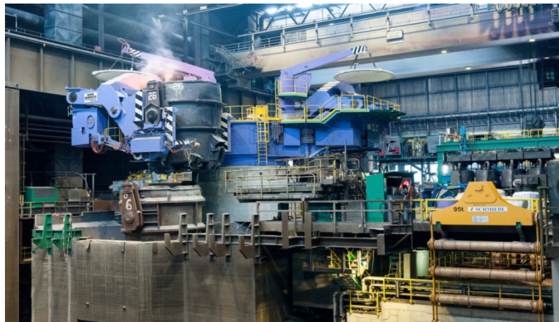
Figure 1. The new ladle turret and casting platform
