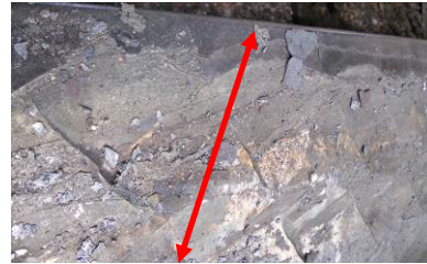
Example of good scarfing showing flat transition near the slab edge. Note the overall smoothness across the scarfing.
