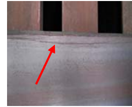
Example of plate edge defects that can be created by poor scarfing technique
