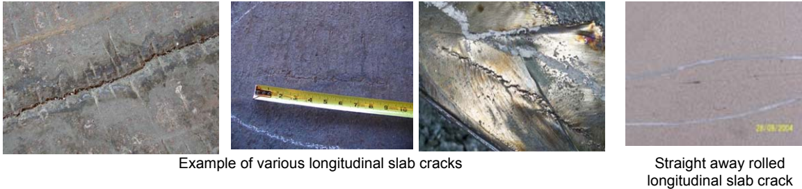
Figure 2. Example of longitudinal slab cracking.
