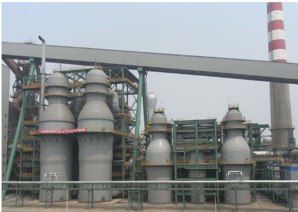
Figure 4. KSS systems of BF No. 1 and No. 2 with capacity of 5,500 m 3 in Shougang Jingtang United Iron and Steel Co., Ltd., blast temperature of 1,300°C with combustion air up to 570°C in small KSS.
