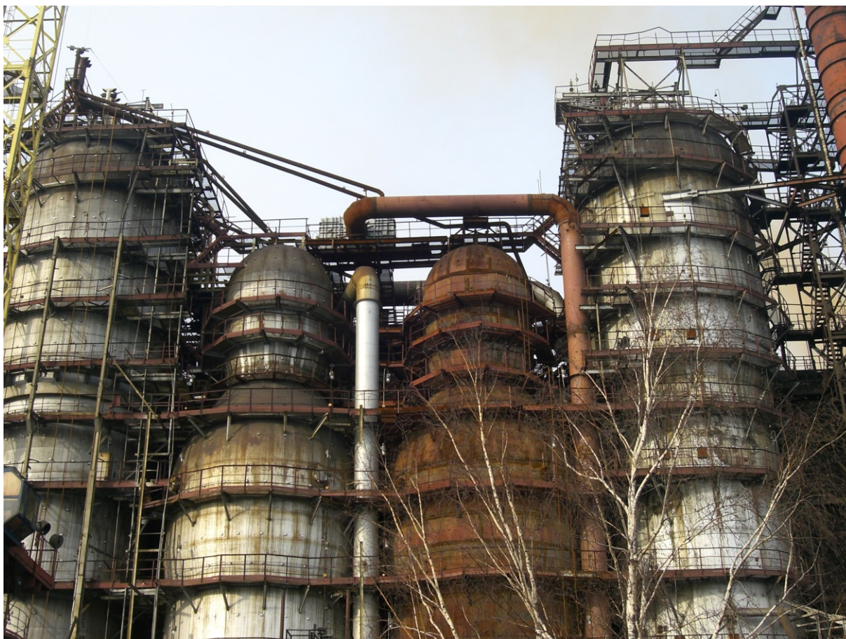
Figure 5. 2 KSS between in internal hot stoves of .№1 BF 3000 m 3 in OAO ZSMK in Russia
