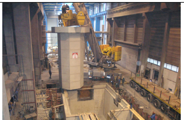
Figure 2: installation works of biggest vertical centrifuge of the world at IRLE in Netphen-Deuz, Germany.
