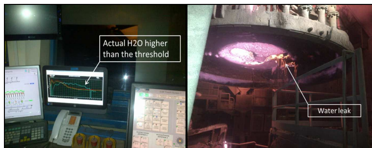
Figure 14: High Warning for water leak generated on EAF operator screen
