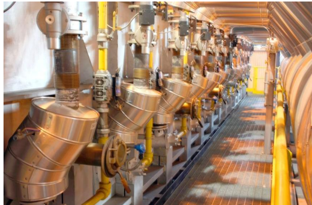
Figure 6: Austenitizing Furnace, digitally controlled burners battery
