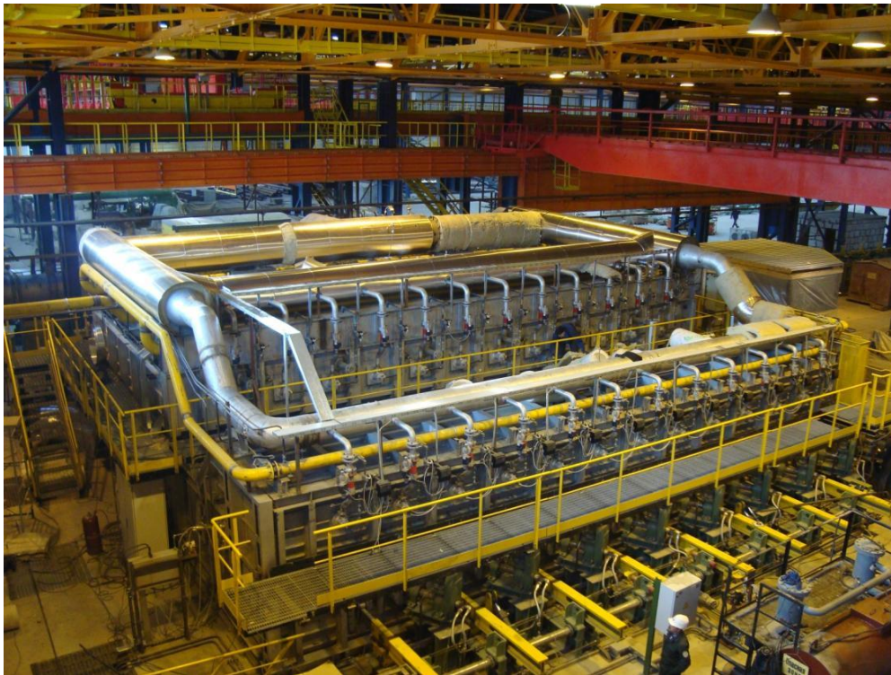
Figure 8: Austenitizing Furnace, aerial view.
