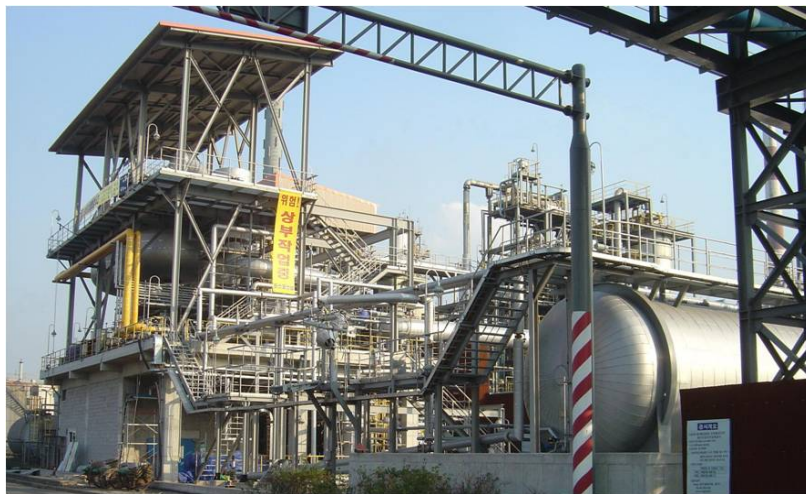
Figure 3. Claus plant in Asia.
