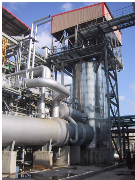
Figure 4. Burner and boiler unit.
