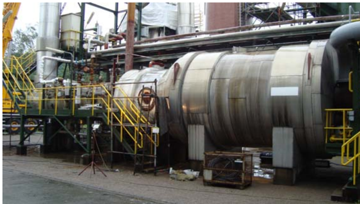
Figure 8. Old combustion unit with waste heat boiler.
