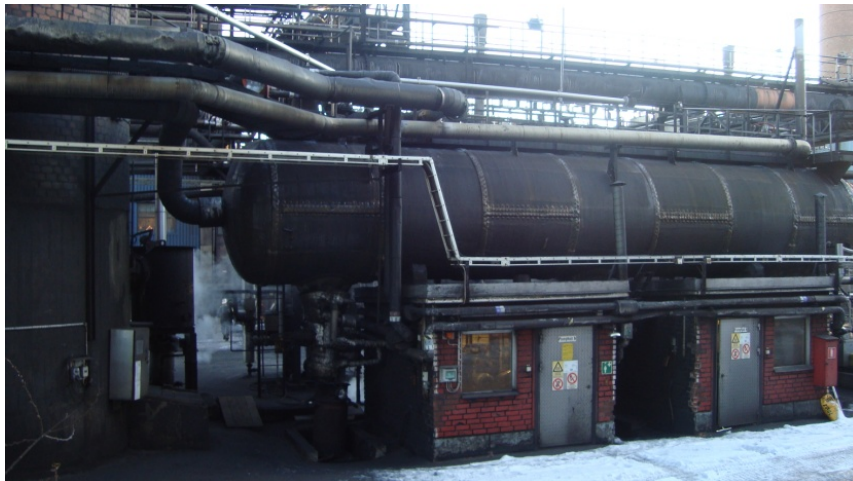
Figure 1. Old tar separation unit.
