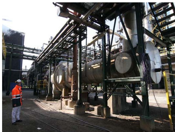
Figure 9. New combustion unit with waste heat boiler.
