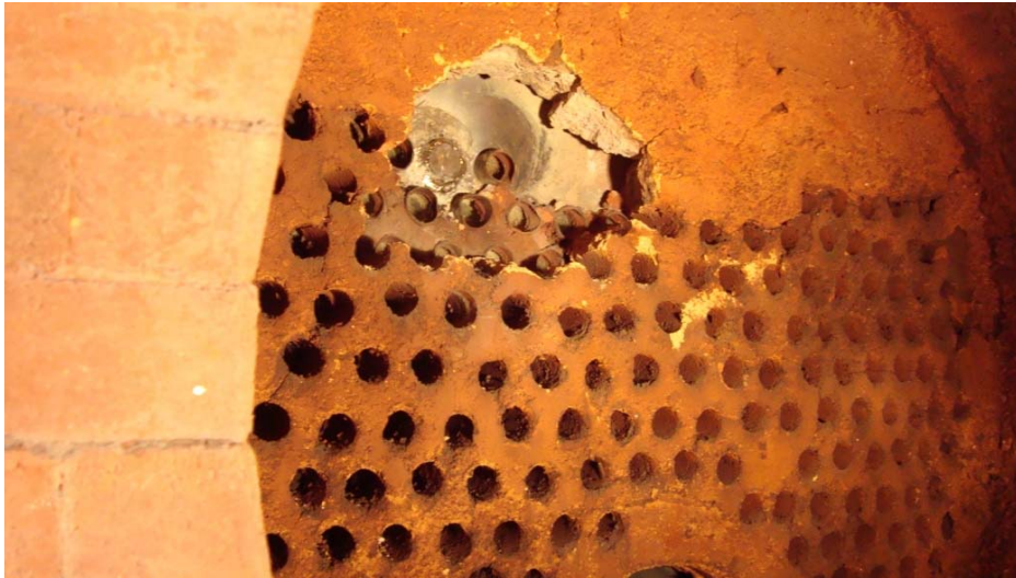
Figure 10. Broken lining inside waste heat boiler.
