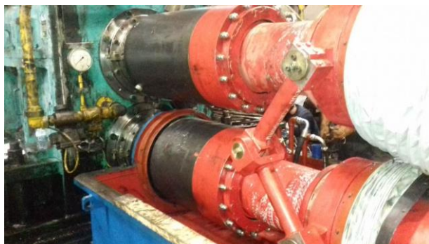
Figure 20. Spindles and Anti-rotation Device Installed
