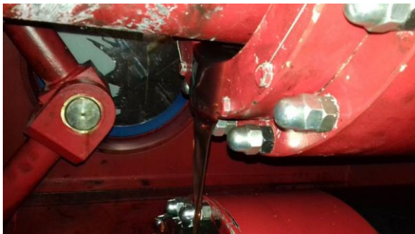
Figure 24. Oil Discharge Check
