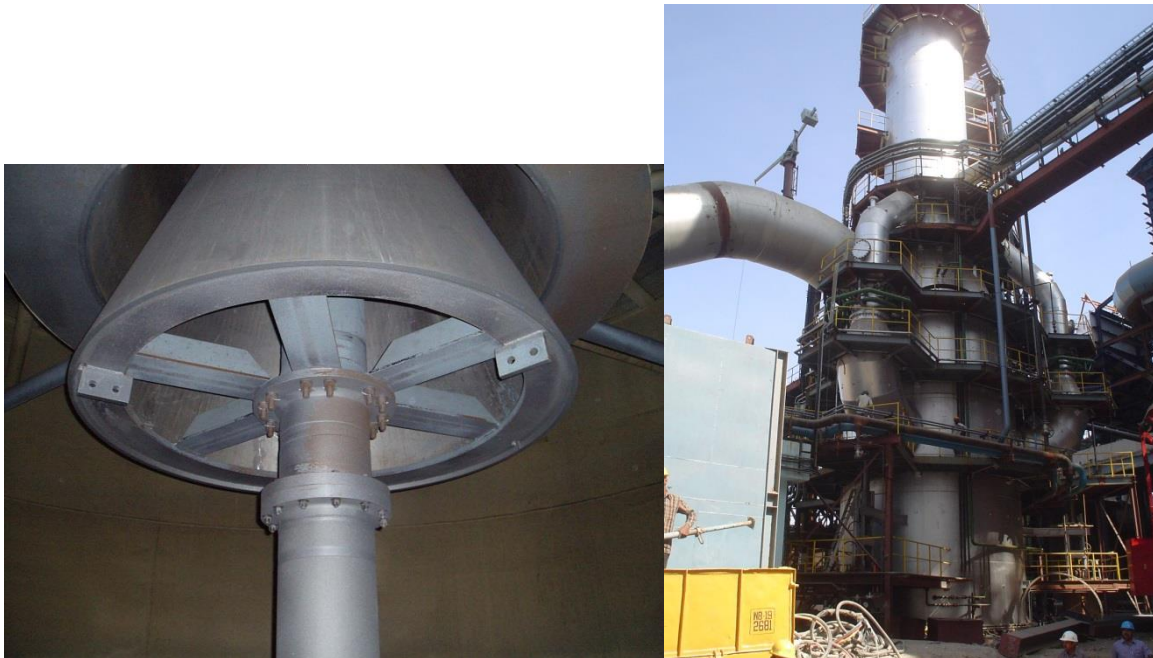
Figure 4. View on the cone element from the bottom (left) & scrubber installation with external cone elements (right).
