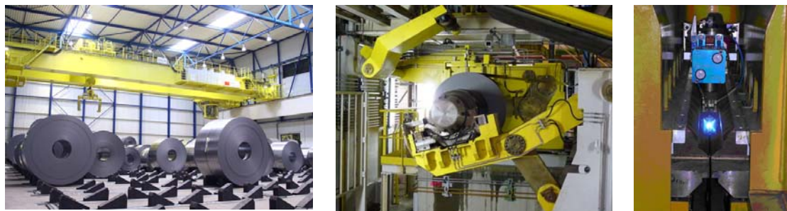
Figure 1. Entry coil storage area, pay-off reel and laser welder.
