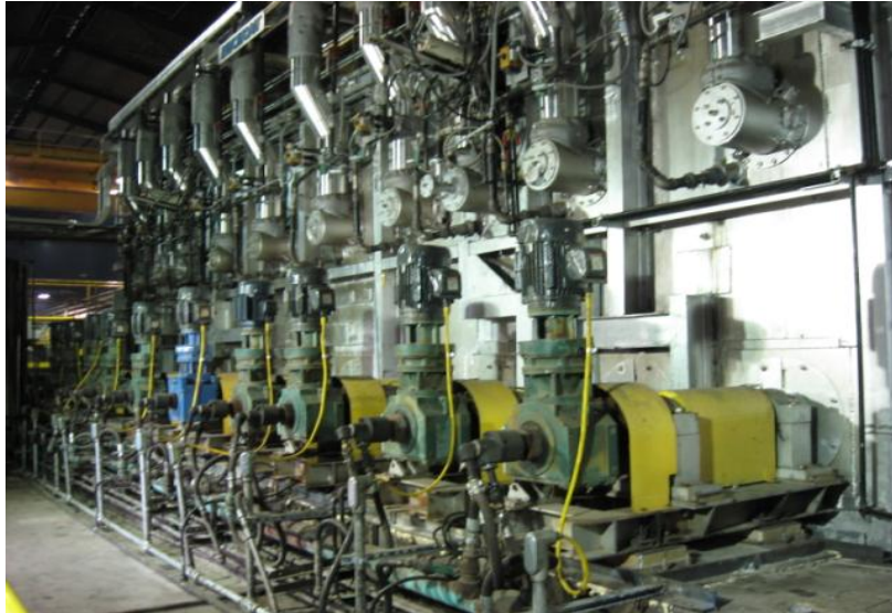
Figure 2: Discharge End of New Furnace
