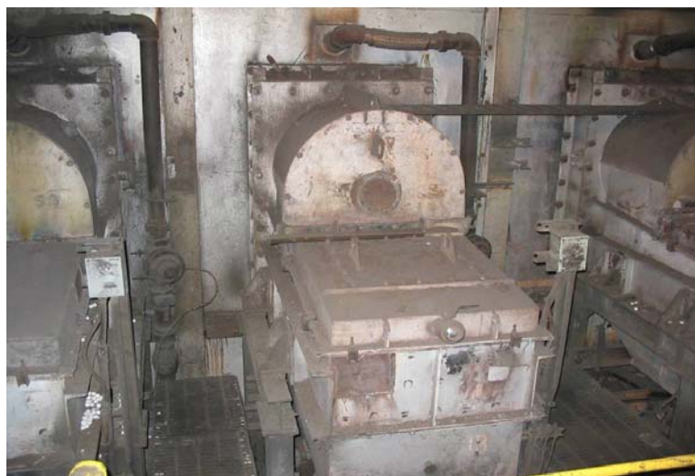
Figure 10: Existing Regenerative Burner
