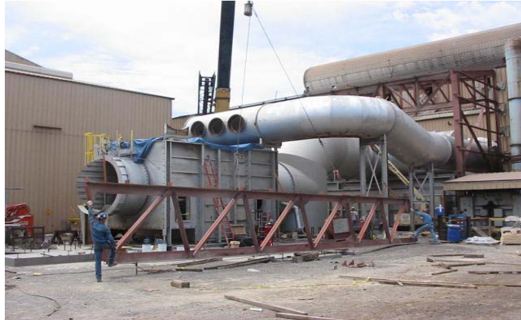
Figure 8: New Recuperator and Combustion Air Piping.
