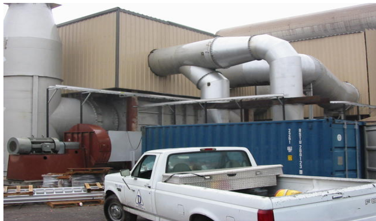
Figure 9: New Ejector Stack
