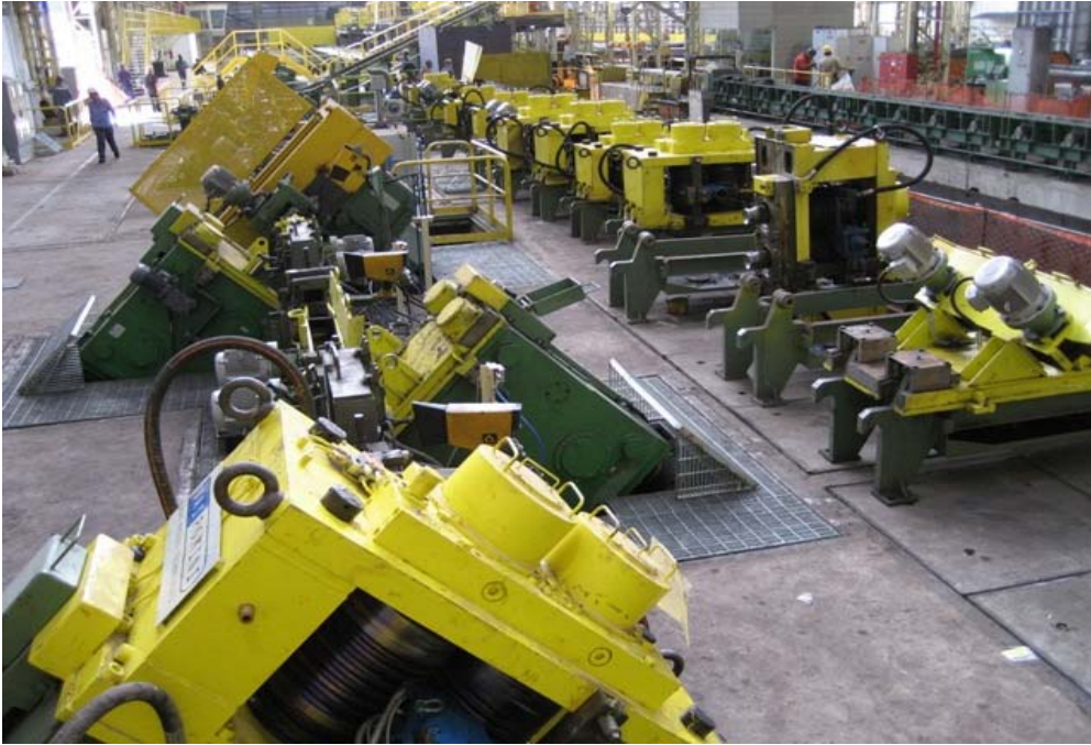
Figure 4 - CCR (Cassette-type Compact Rolling) Stands and Standby Cassettes
