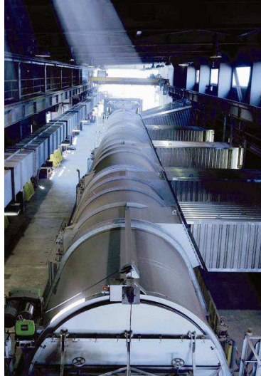
Figure 7: Hooded sinter strand at voestalpine Linz/Austria showing offgas recirculation ducts to the right.
