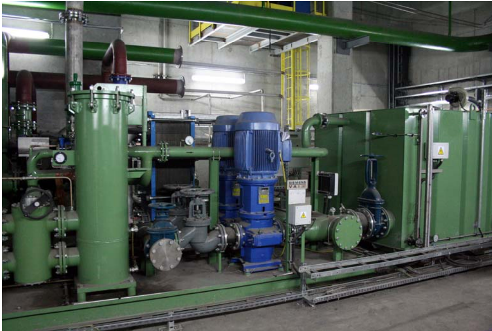
Figure 1. Full single tank lube system on two pallets.
