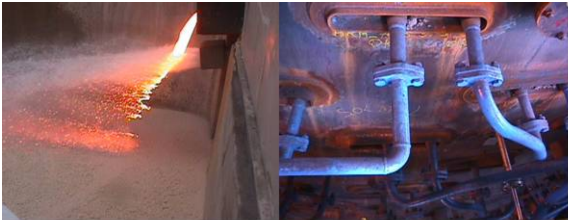
Figure 5: New slag granulation in operation and new pipes for the BF cooling system.
