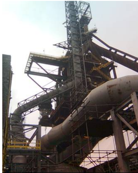
Figure 6: BF1 overview with new slag granulation chimney.
