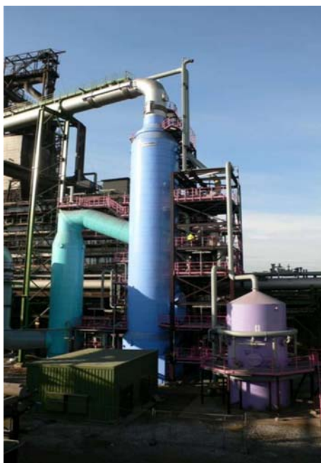
Fig. 10: BF Gas scrubber at ThyssenKrupp’s BF No.8
