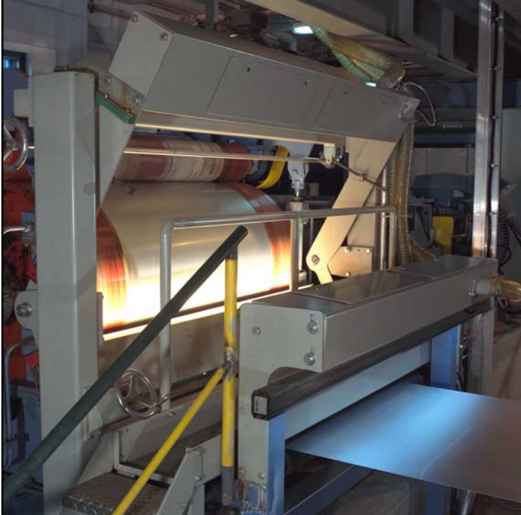
Figure 3. ABB SIS installed on annealing and pickling line in Outokumpu Tornio Works in Finland.
