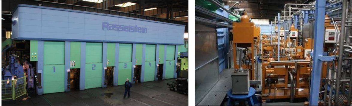
Figure 9: TCM Rasselstein after revamp with new cladding (l) and new service platform (r)
