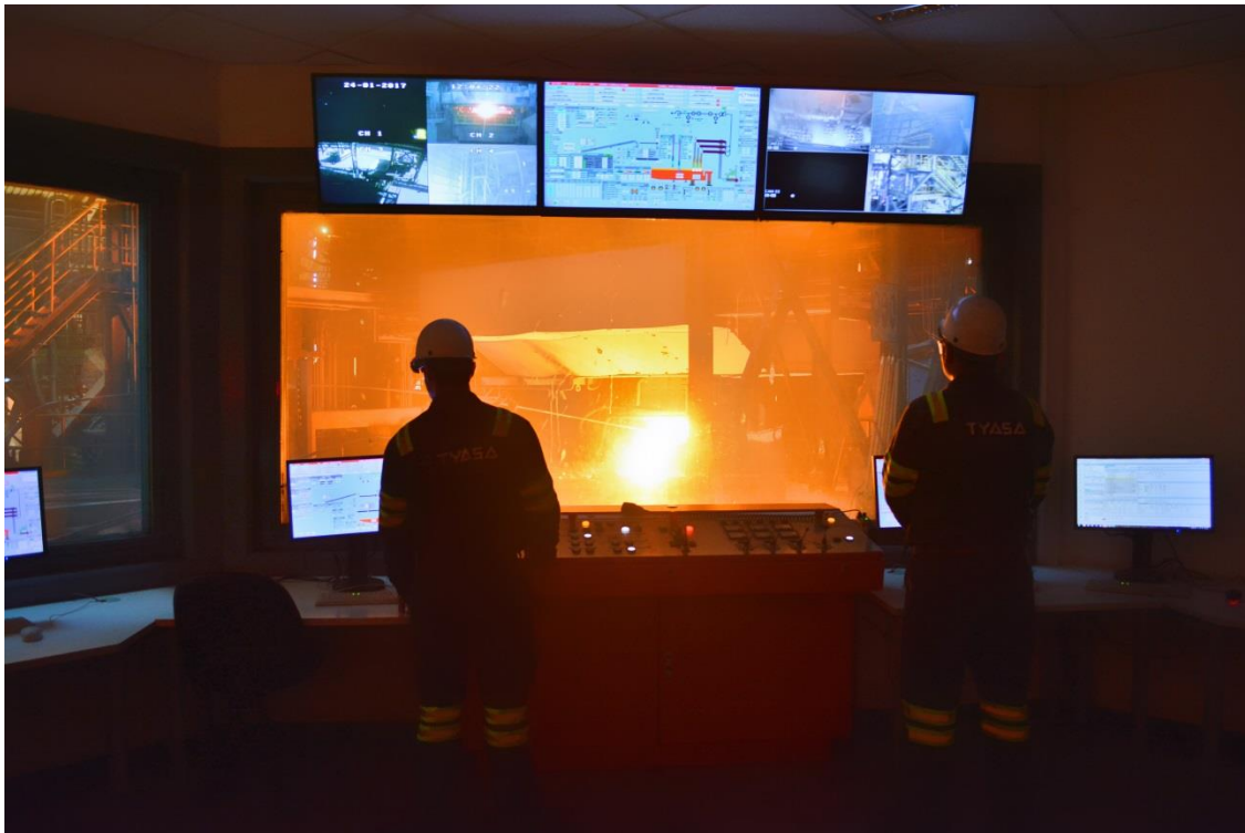
Control pulpit in Tyasa's plant in Ixtaczoquitlan, Mexico. (Photo courtesy of Tyasa).
