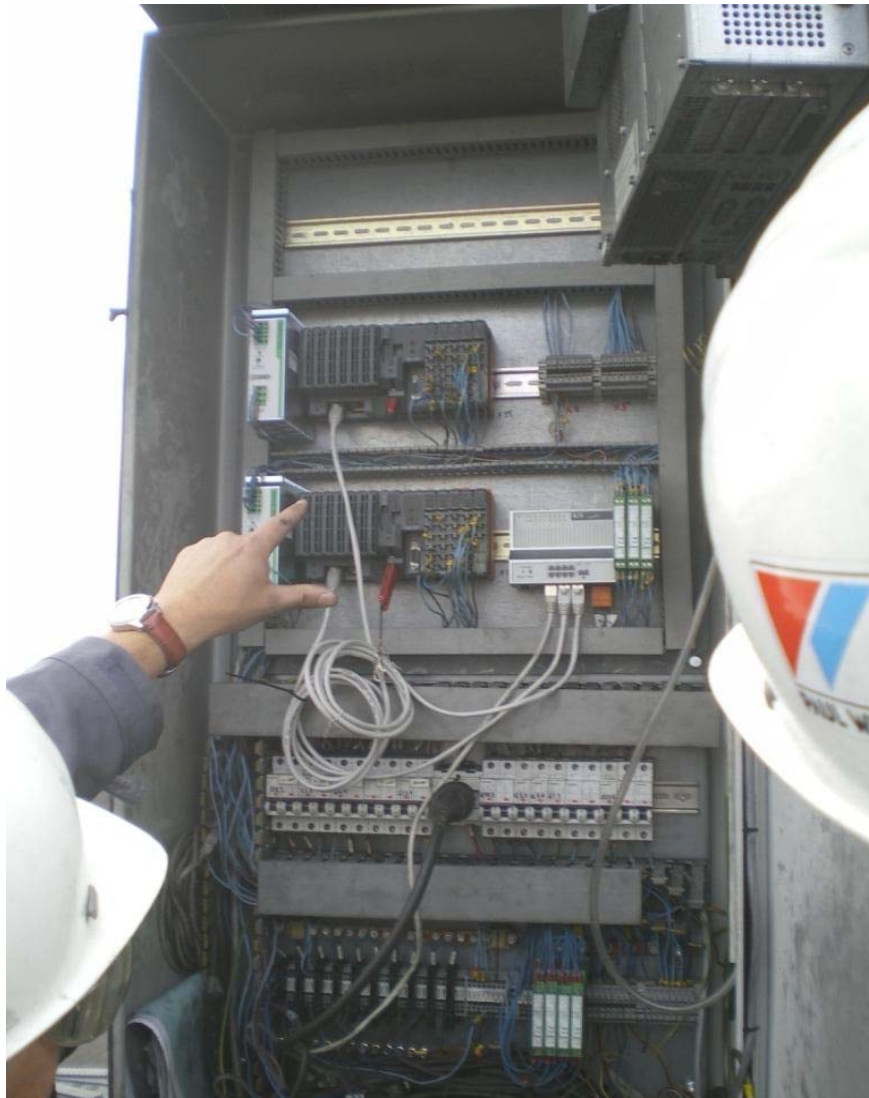
Figure 5. Control Panel for Sopreco ® valve Trial.
