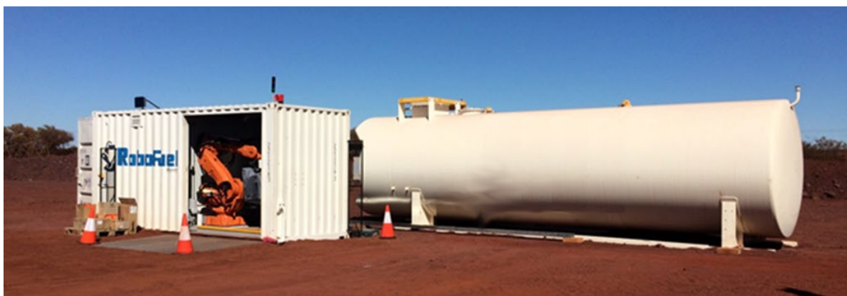
Figure 7. Robofuel installed in-pit, with modular container, pumping and power for remote operation
