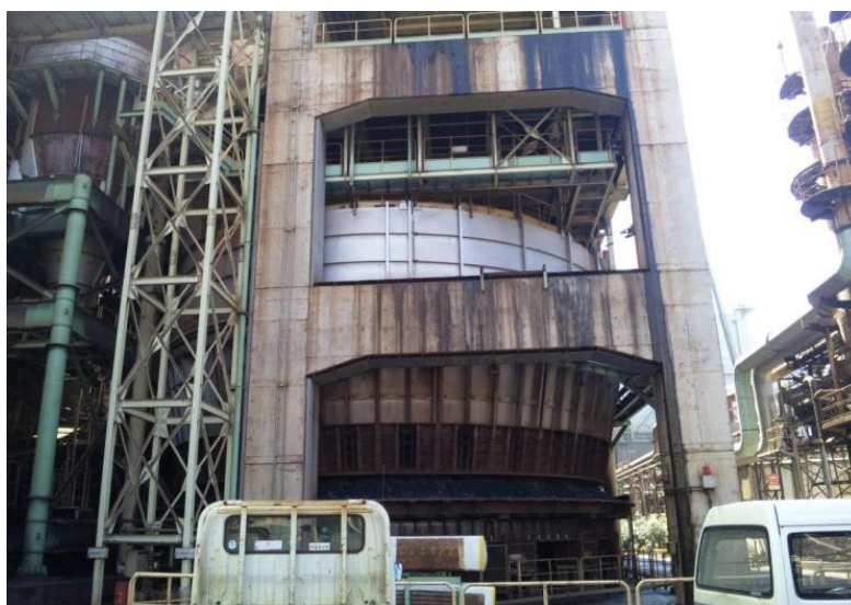
Figure 3. Circular hopper cooler installed at NSSMC Wakayama No.5 sinter plant.
