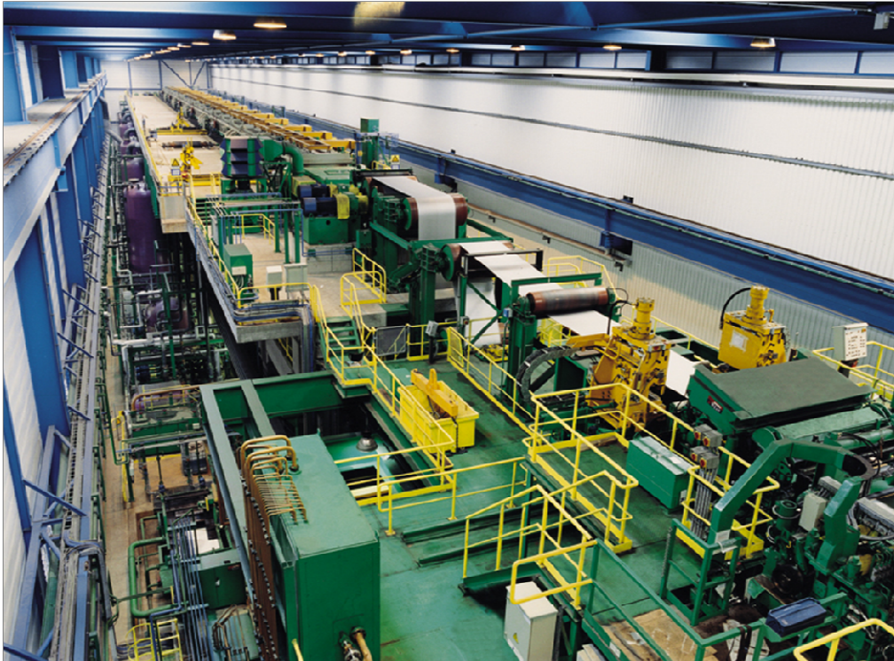
Figure 2 – Overview of entry side of pickling section.
