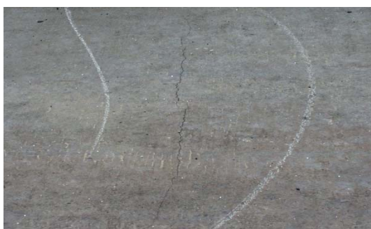
Figure 12. Transverse crack of slabs.
