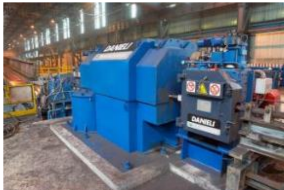
Figure 6. The HSS-High Speed Shear in operation at Ferriere Nord – Italy.
