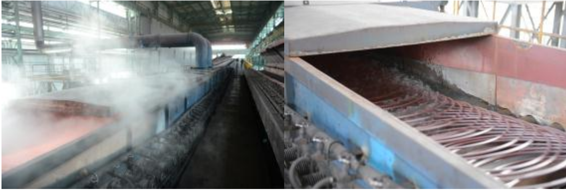
Figure 9A and 9B. EDC system in operation at Angang Anshan I&S – P.R. of China
