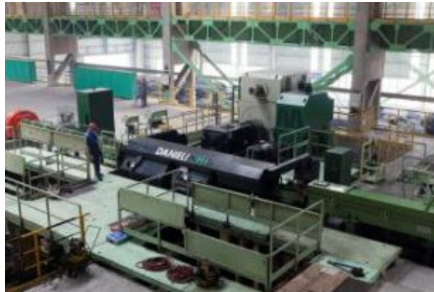
Figure 5. The Twin Module Block in operation at Zhangdian I&S – P.R. Of China.
