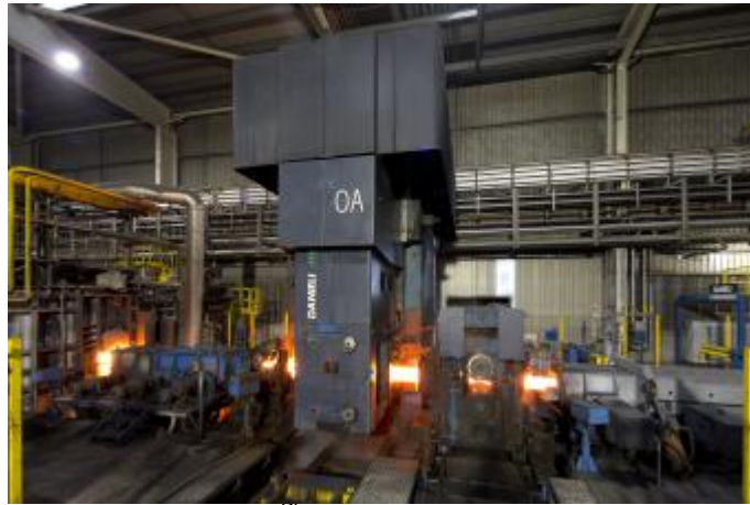
Figure 2. SHS Plus in operation at ABS – Italy.
