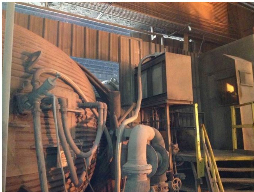
Figure 2: Heated Line on a Down-stream location
