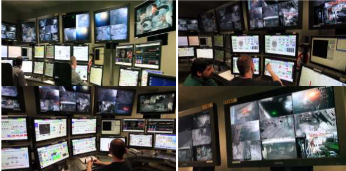
Figure 1 - The Modern EAF control room with no exposed windows to the EAF or operating floor
