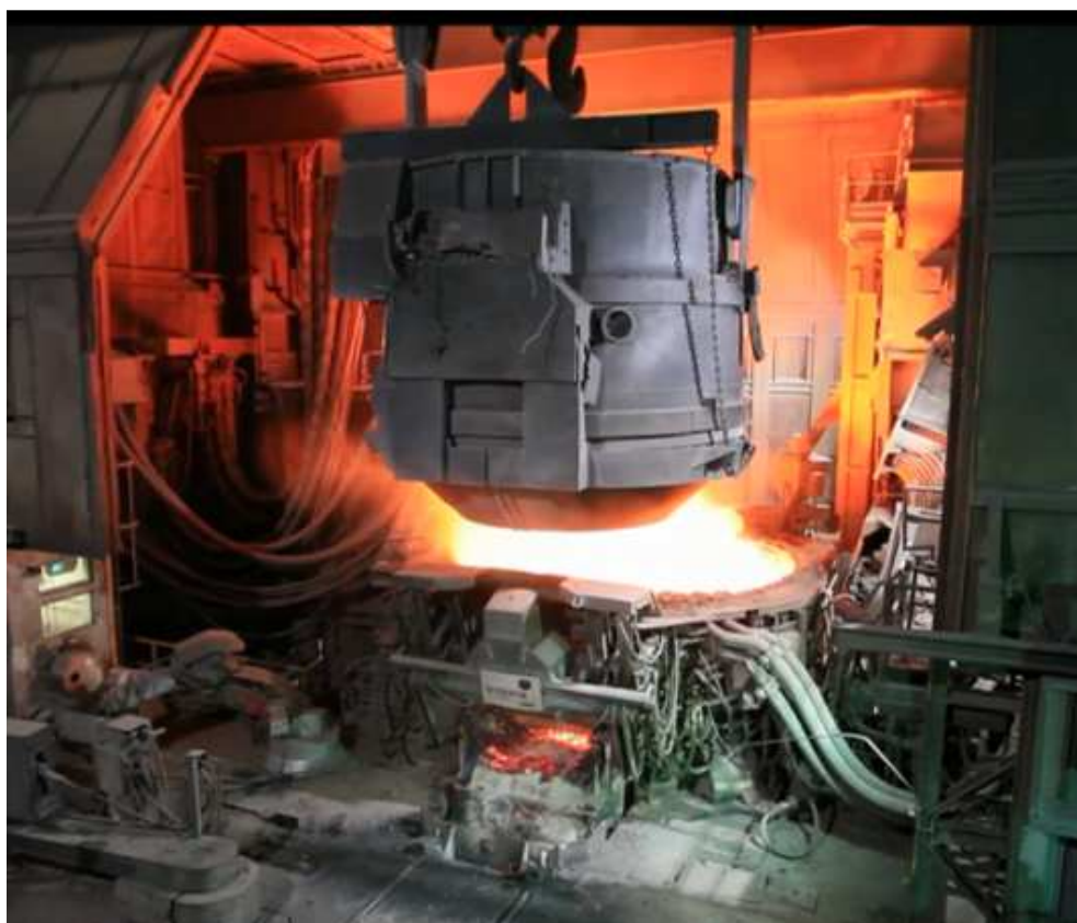
Figure 15. Scrap bucket automatically charged to the EAF without the need of a crane operator
