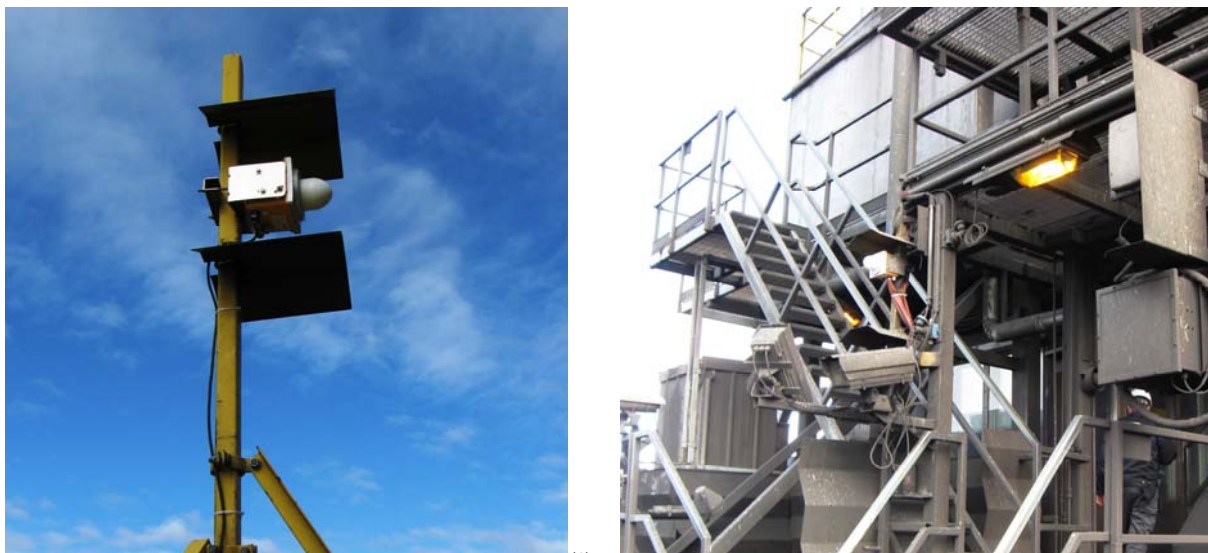
Figure 2. Static- and onboard radar installation. (1)
