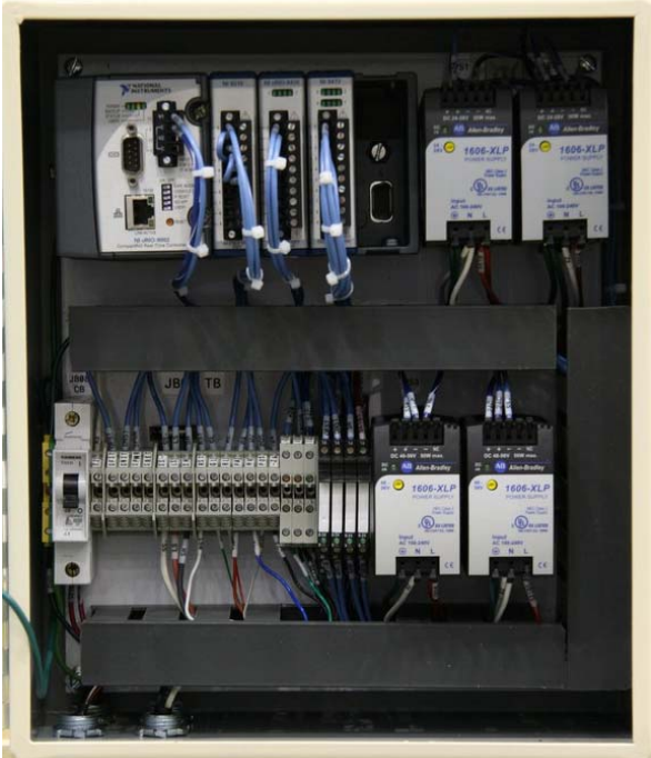
Figure 3 – Photograph of a typical National Instruments cRIO PAC and associated equipment.
