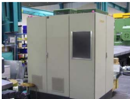
Figure 8. Energy box at assembly site
