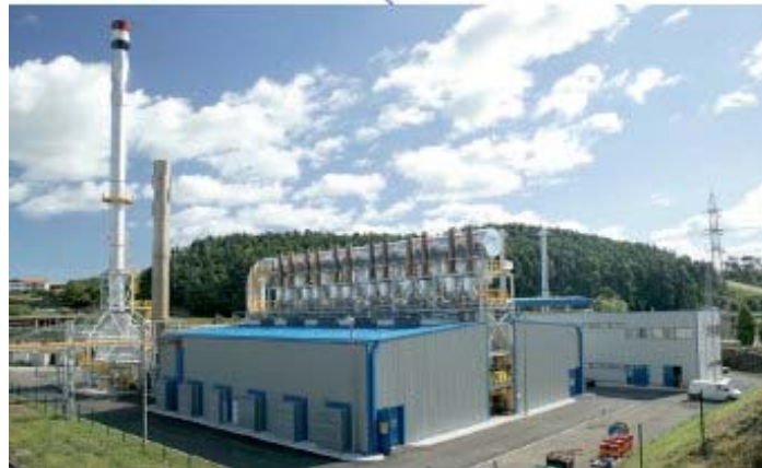
Figura 6: Power house 12 x J620GS; 20.4Mwe
