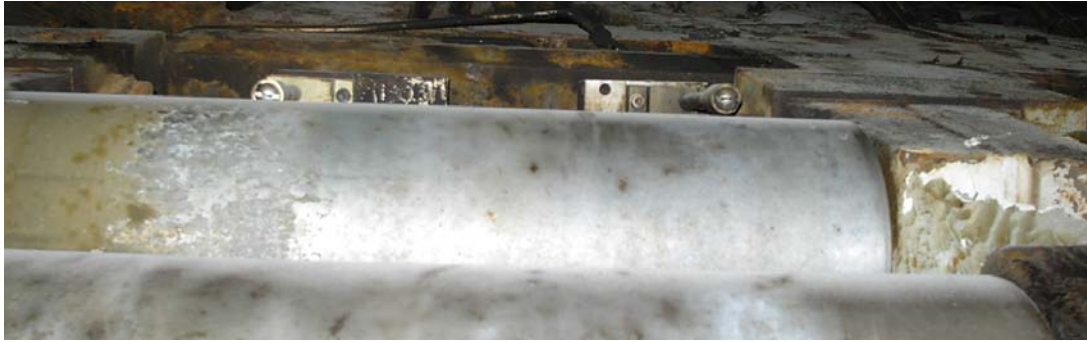
Figure 5 – Misaligned and off position air mist nozzles.
